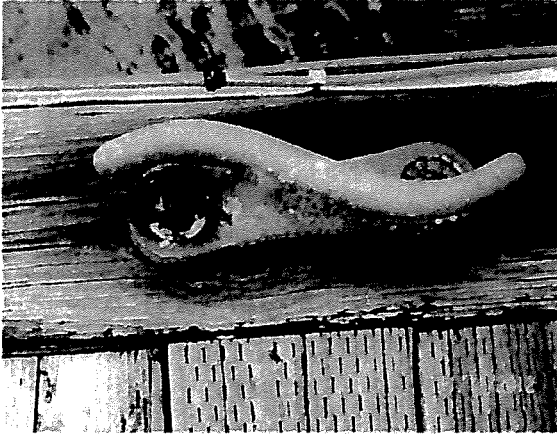
Figure 18: Rusty, missing mounting bolts.
