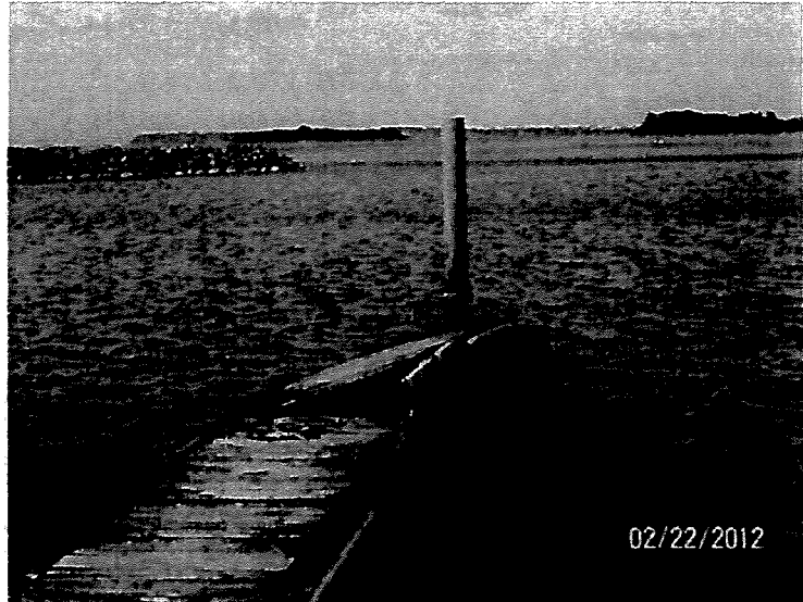
Figure 26: Pier D finger pier damage. Note the date of this photograph. This finger pier remains unrepaired at the date of this essay, November 12, 2012.
