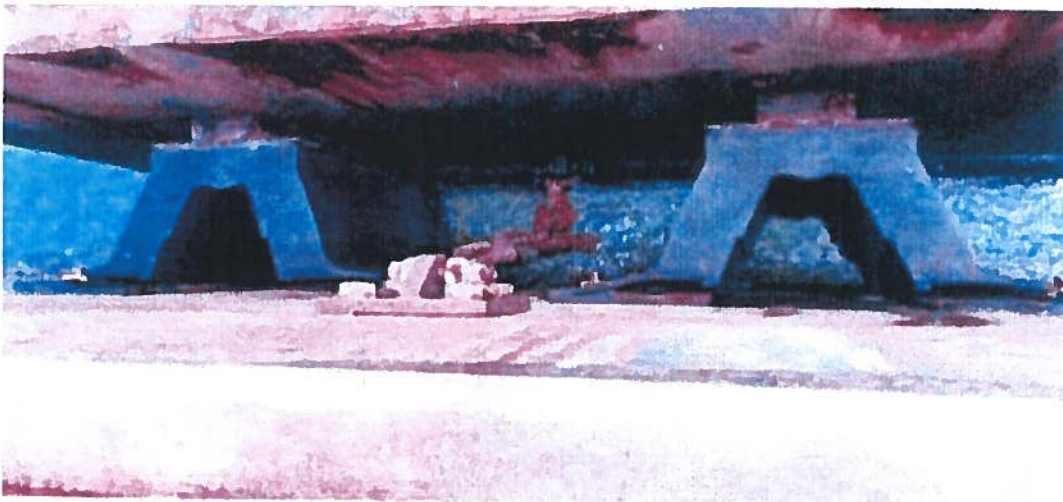
BERTH F5 DAMAGED RUBBER LEG ARC FENDER
