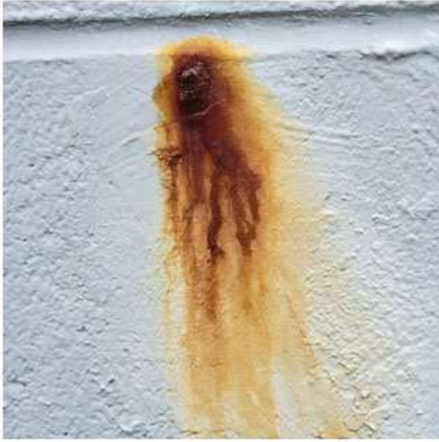
Figure 7 Example of Rust Stains - Damage to be Repaired.
