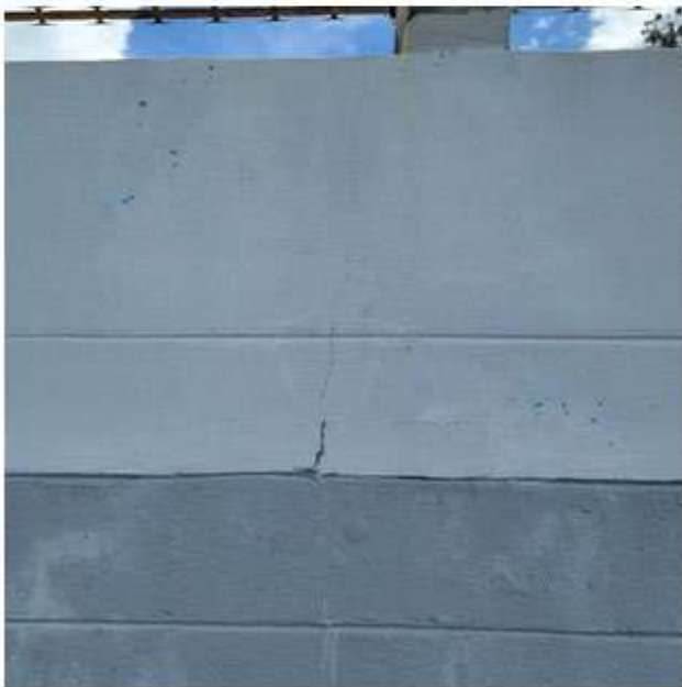
Figure 11 Example of Crack
