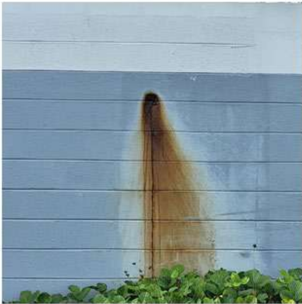
Figure 9 Example of Rust Stains - Damage to be Repaired.
