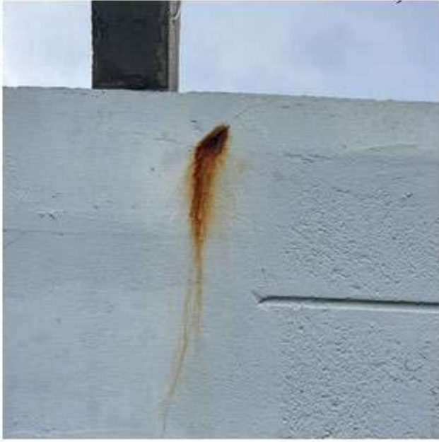
Figure 8 Example of Rust Stains - Damage to be Repaired.
