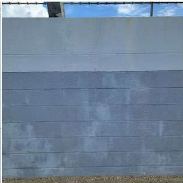
Figure 12 Example of Crack
