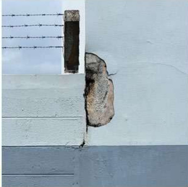
Figure 2 Load Center 4 Concrete Damage
