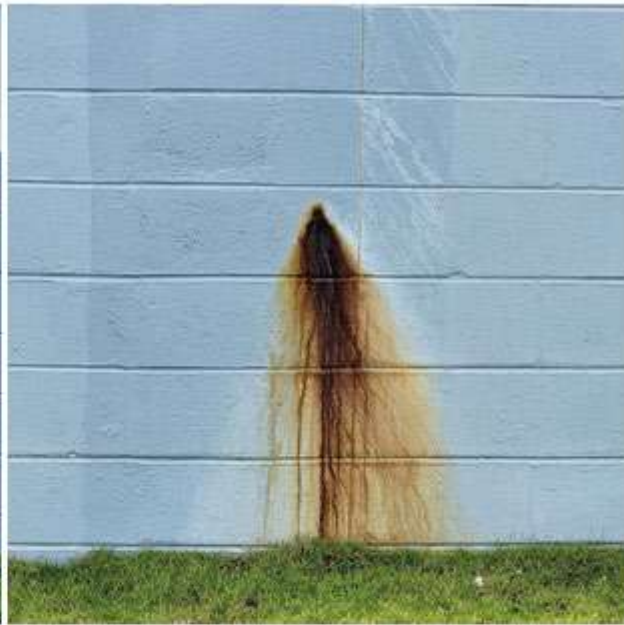
Figure 10 Example of Rust Stains - Damage to be Repaired.
