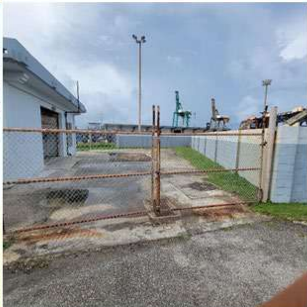
Figure 4 GWA Pump Station Bldg. – Wall inside gate to be painted
