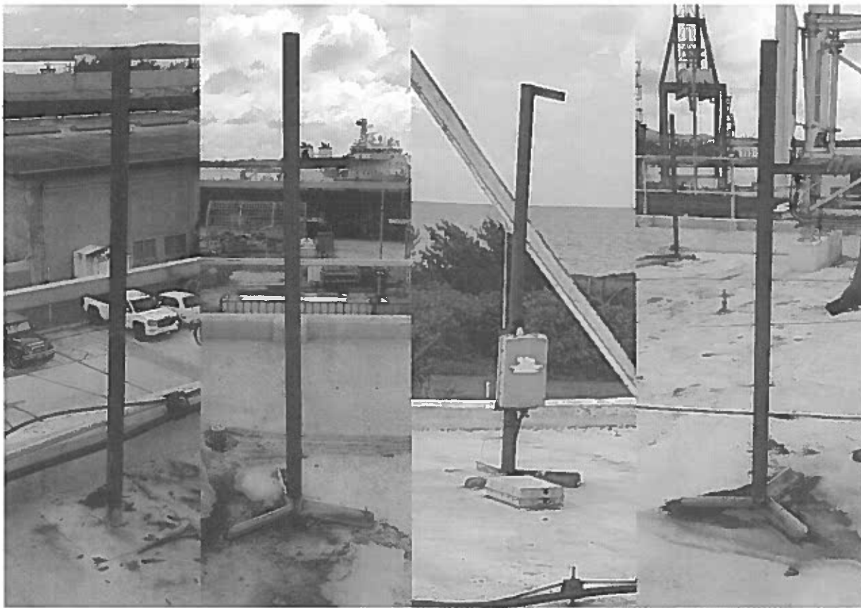
Figure 3: Surface Mounted Steel Pipes
