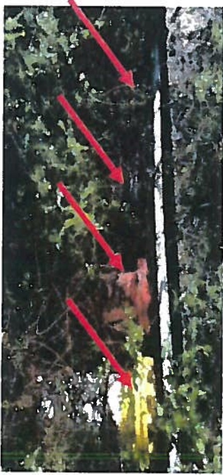
Station 02+69 Replace Corroded Bolts/Nuts & Paint all Flanges
