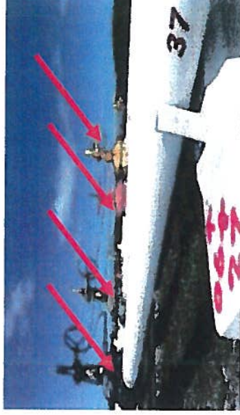
Station 06+27 Corrosion At All Gate Valves
