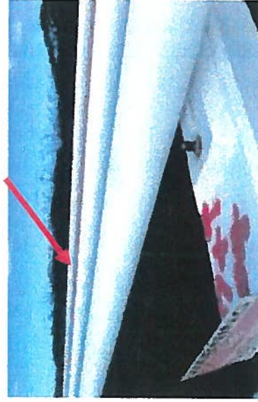
Station 07+04 Corrosion of Fire Saltwater Line
