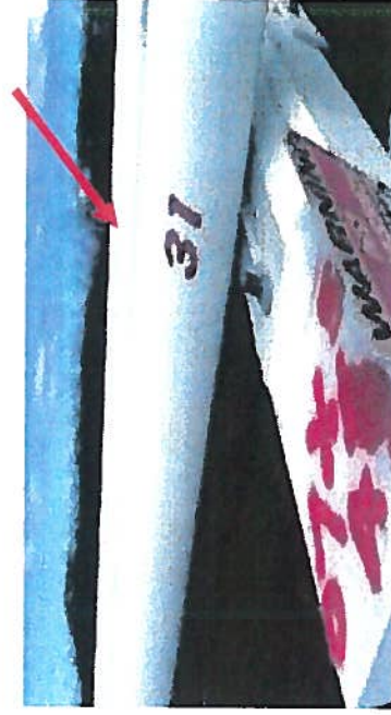
Station 07+45 Corrosion of Fire Salt Waterline
