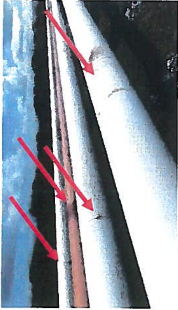
Station 04+63 Corrosion of All 4 Pipelines
