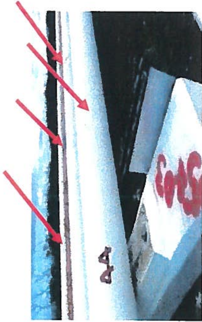
Station 05+03 Corrosion At All 4 Pipelines
