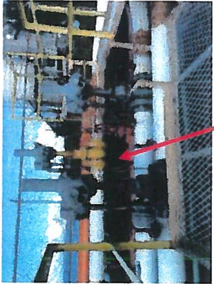
Station (00+00) Valve Pit Area Inside Mobil Facility
