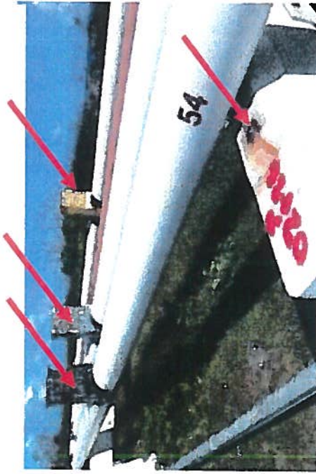
Station 02+86 Re-paint 3ea Screen, Gate Valve and corroded nut
