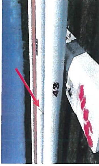
Station 05+16 Corrosion At Jet Fuel Pipeline
