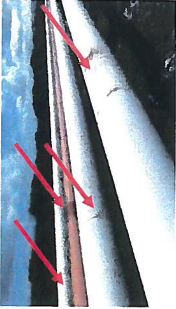
Station 05+44 Corrosion At All Pipelines
