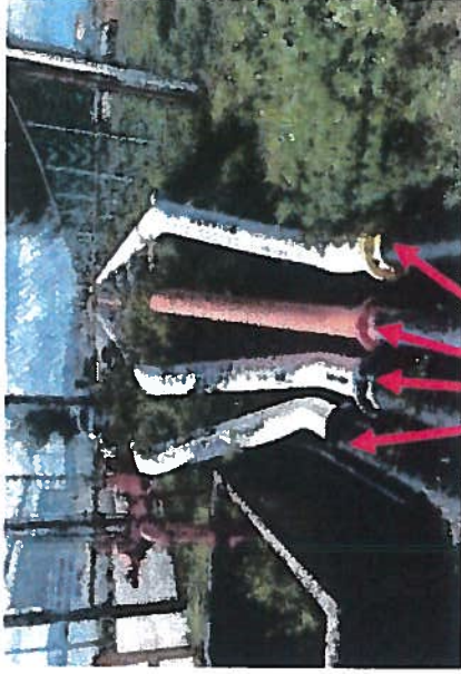
Station 02+15 Replace Corroded Bolts-Nuts Re-Paint All Pipeline Flanges
