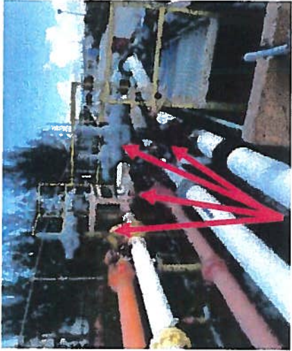
Paint the Three Corroded MOV Valves and the Fire Saltwater Line Gate Valve
