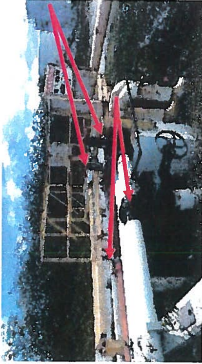
Replace Corroded Bolts/Nuts As Required. Paint Corroded Flanges and Gate Valves
