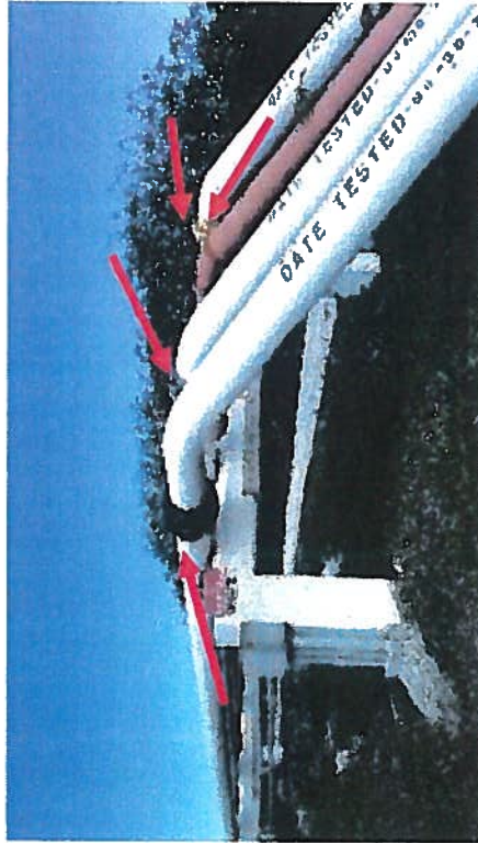
Replace Corroded Bolts & Nuts as Required & Repaint All Flanges and Corroded Pipeline
