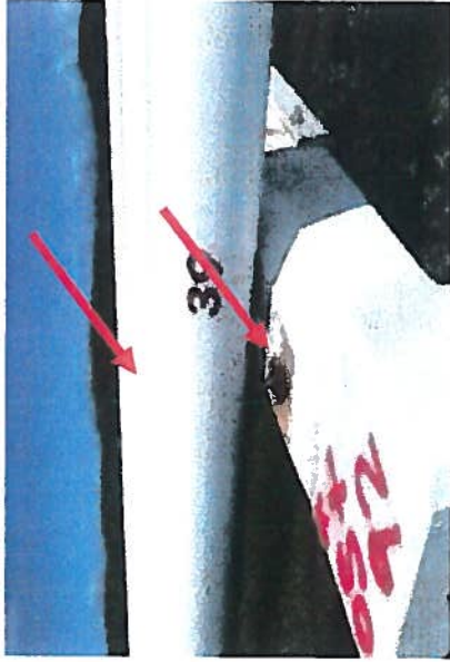
Station 05+92 Corrosion of Jet Fuel Pipeline and Replacement of Corroded nut
