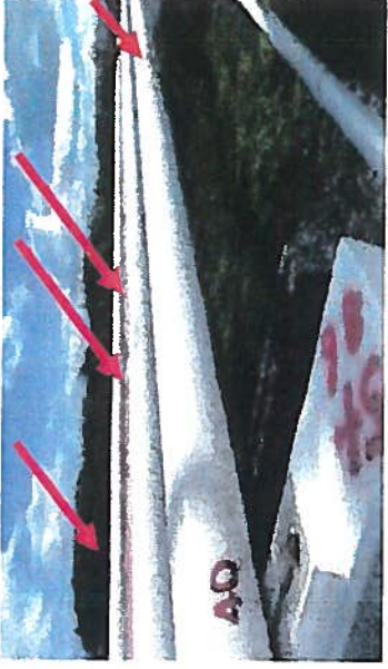
Station 05+86 Corrosion of All 4ea. Pipelines
