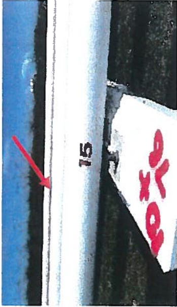
Station 10+76 Corrosion of Fire Salt Waterline
