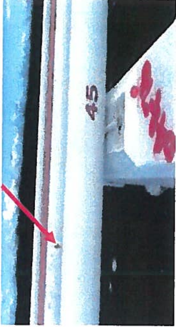
Station 04+76 Corrosion of Jet Fuel Pipeline
