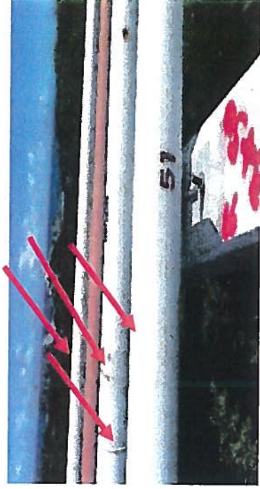
Station 03+50 Corrosion of All 4 Pipelines
