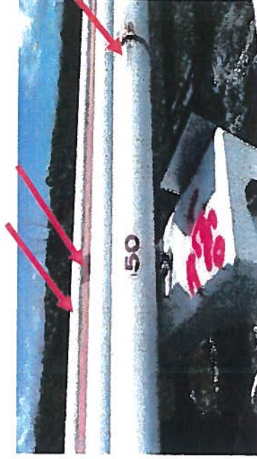
Station 03+79 Corrosion of 3ea. Pipelines
